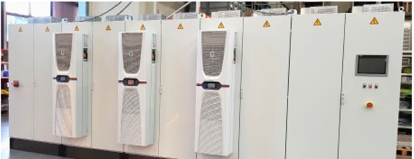
Just a part of the bigger picture: the large dimensions of the cleaning system conceal a high degree of technical sophistication.
