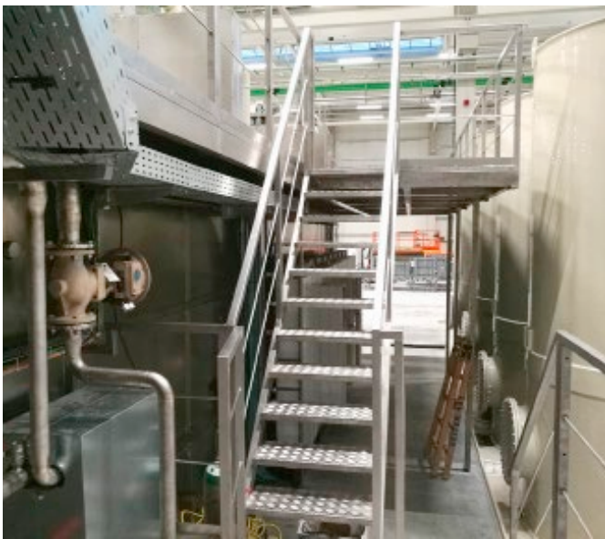
Secure access to the top of the plant ensures it can be fully serviced.
