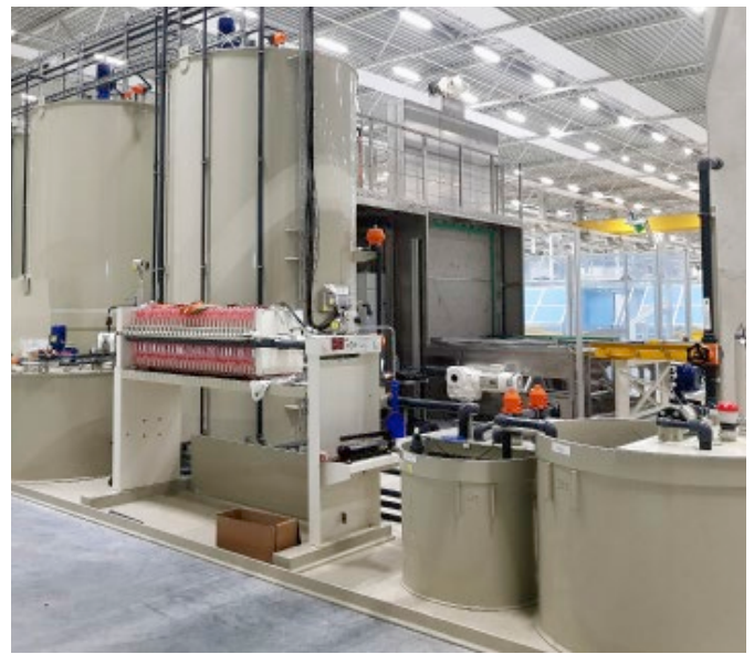
A separate water treatment plant ensures that the waste water is chemically and physically treated so that it can be discharged into the public drainage system.
